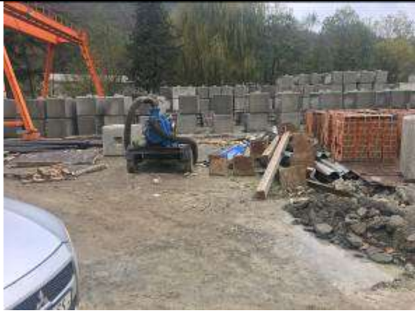
Workers without PPE, power generator without drip tray
